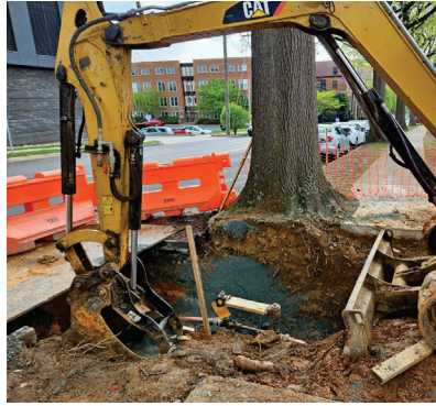
Tree Preservation, Garrett St. Mature Tree Damage
